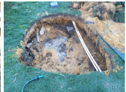
Not removing or decommissioning a septic tank
