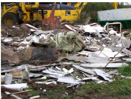
Inappropriate disposal and removal of asbestos cement material
